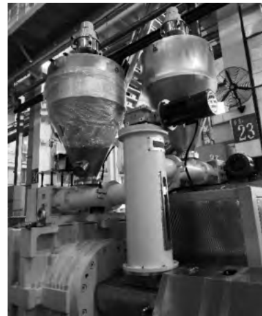
Figure 2 Material conveying system
