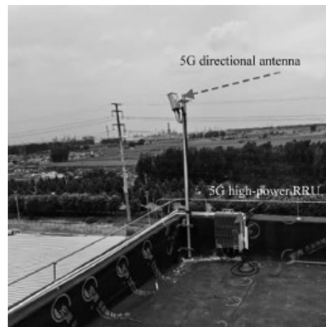
Figure 2 5G high-power RRU and directional antenna deployed on the rooftop
